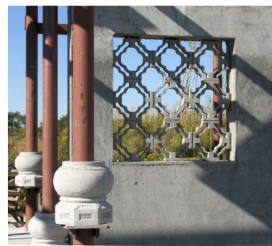
Perforated 'Leak Window' in Knowing the Spring Pavilion
